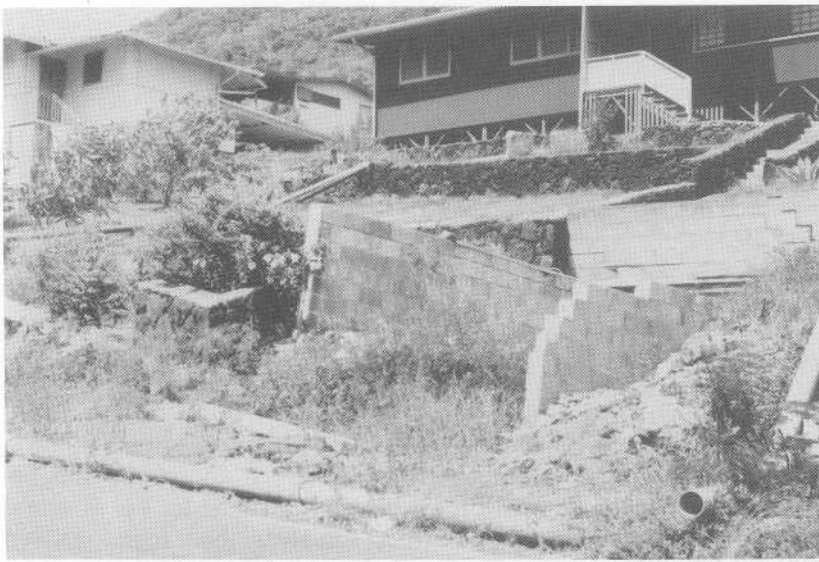
FIGURE 18.28 Structural failure caused by landslide on Vertisols produced by wet soil sliding downhill. Note that pipes are on top of the ground to prevent breaking caused by expansion and contraction of soil.
