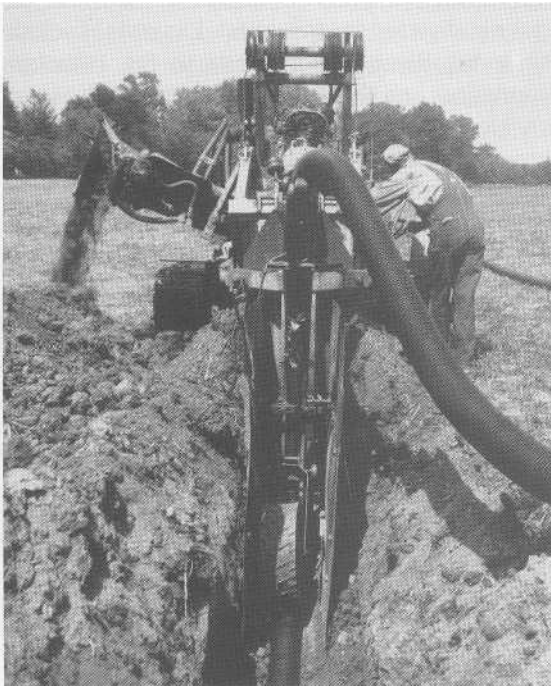
FIGURE 6.7 Installation of perforated plastic tubing to remove water from a field during the wet season. The plastic tubing carries water to an outlet where the water is disposed. (Photo courtesy Soil Conservation Service, USDA.)
