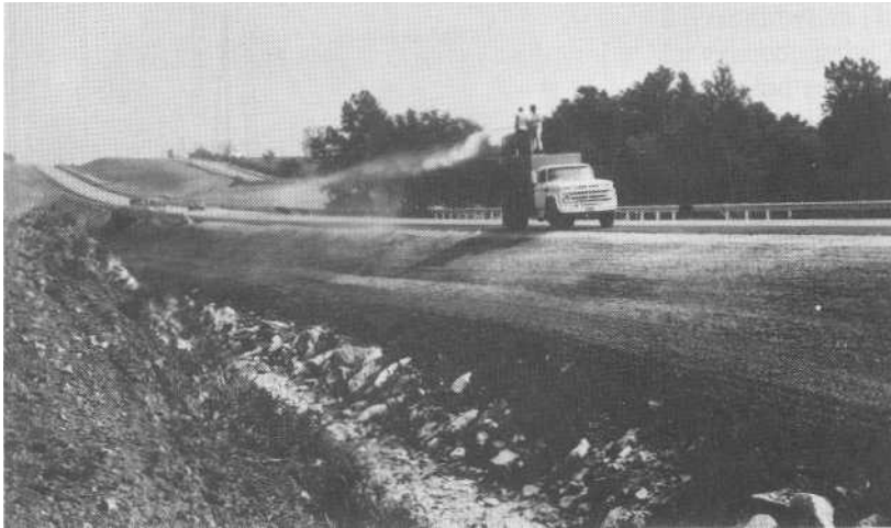
FIGURE 7.11 Slurry truck spraying fertilizer and seed on freshly prepared seedbed along road in Missouri. A thin layer of straw mulch will be secured with a thin spray of tar to protect the soil until vegetation becomes established. (Photograph courtesy Soil Conservation Service, USDA.)
