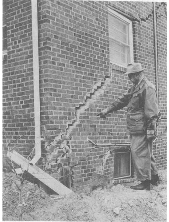
FIGURE 3.5 Foundation soil with high clay content expanded and shrunk with wetting and drying, cracking the wall. (Photograph courtesy USDA.)
